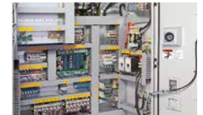
C. Electrical box Neat and clear wiring configuration
